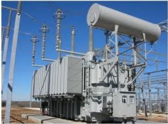
A transformer in a substation.
