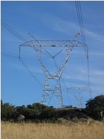
Overhead high-voltage power lines
