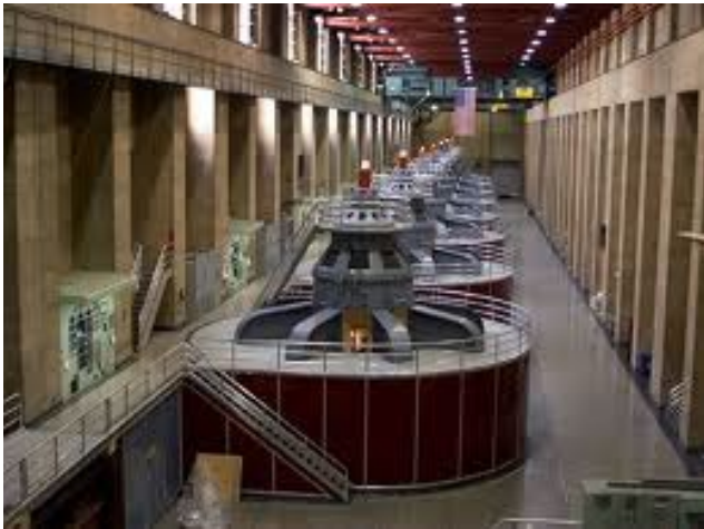
Large AC generators at Hoover Dam.
