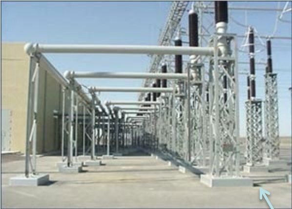
Power buses in a substation.
