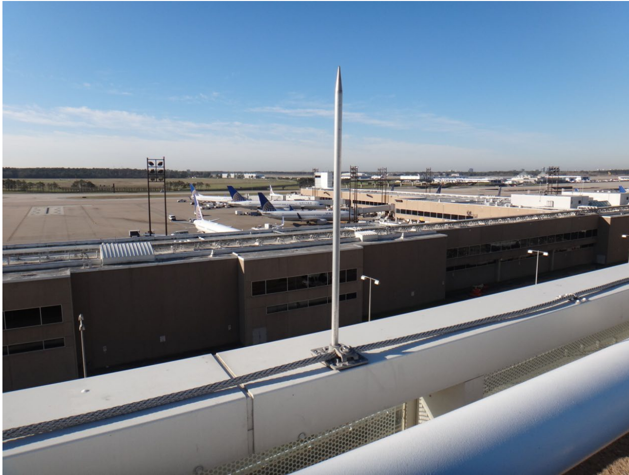
A lightning rod on top of the “Purple Parking Garage” at IAH airport.
