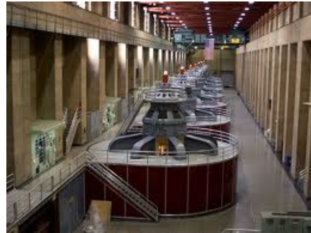
Generators at Hoover dam
