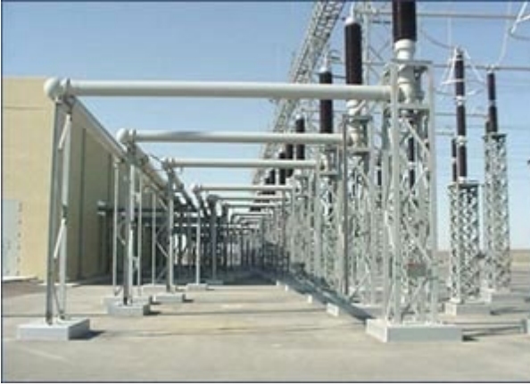
Power buses in a substation
