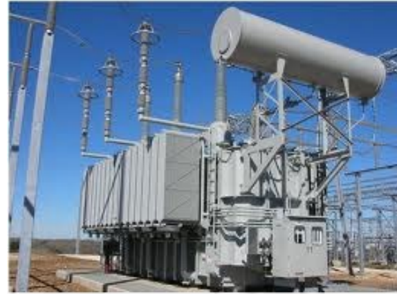
A transformer in a substation
