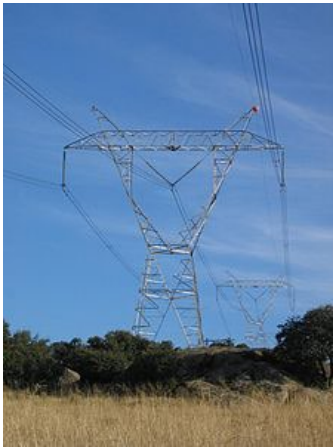
Overhead high-voltage power lines
