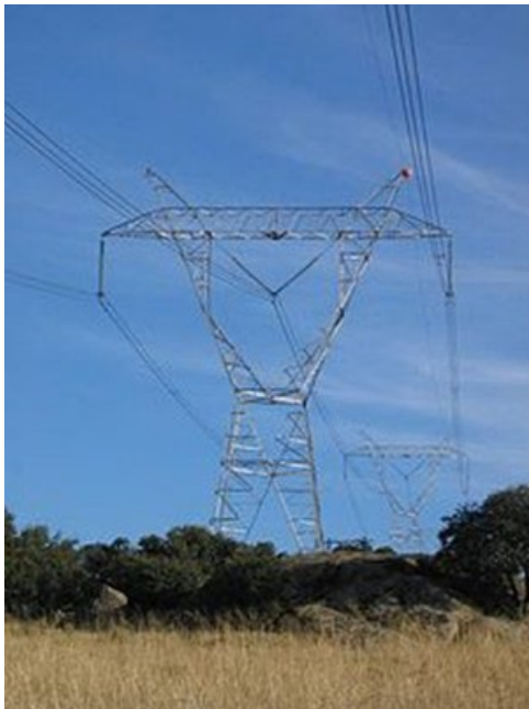
400 kV high-voltage transmission line near Madrid, Spain (Wikipedia)
